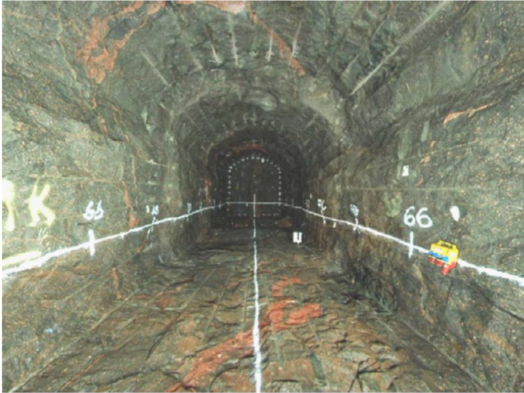
Figure 6-9. A tunnel with a cross sectional area of 20 m 2 was excavated in 2009 at 450 depth in the Äspö HRL. The tunnel is aligned perpendicular to the major horizontal stress and only required spot-bolting support to provide a stable safe opening.
