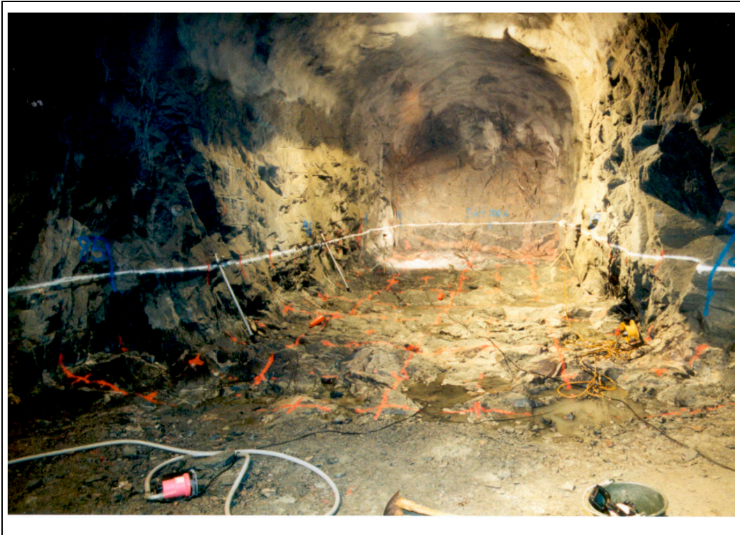
Appendix 3C. Photos showing the tunnel interior. Overview of the entire Canister Retrieval Test Tunnel. Tunnel floor cleaned 2x2m grid-lines marked out Photo: Lars Andersson, SKB.
