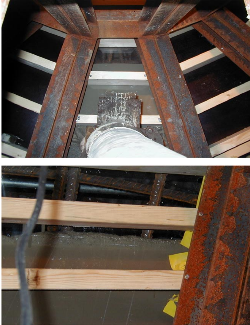
Figure 5-14. The concrete was pumped into the formwork. Lower: The concrete level can be seen through the Plexiglas window. Upper: Pipe connection to the formwork.
