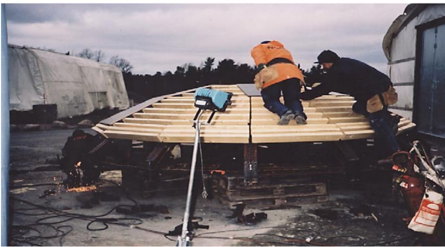
Figure 5-1. The steel is bolted and welded together and crossbars and plywood mounted on the top.
