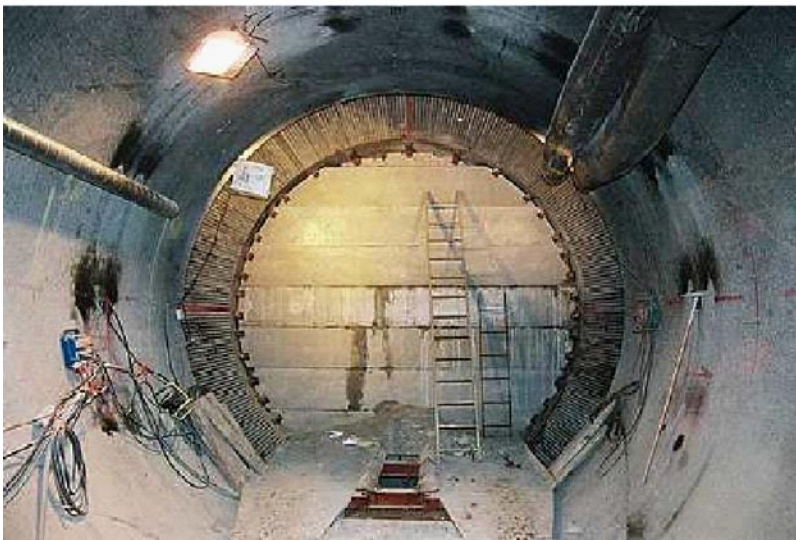
Figure 5-2. The concrete beams are installed successively along with the backfill compaction. The beams are anchored to the rock wall by bolts that are installed in advance of the beam installation.
