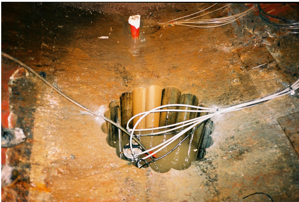
Figure 5-2. The sump and pumps in the inner part of the tunnel.
