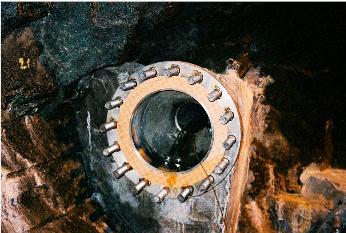
Figure 2-3. Photos showing the installation of steel tubes in the rock (upper) and one completed lead through installed in the rock (without steel flange and cables).
