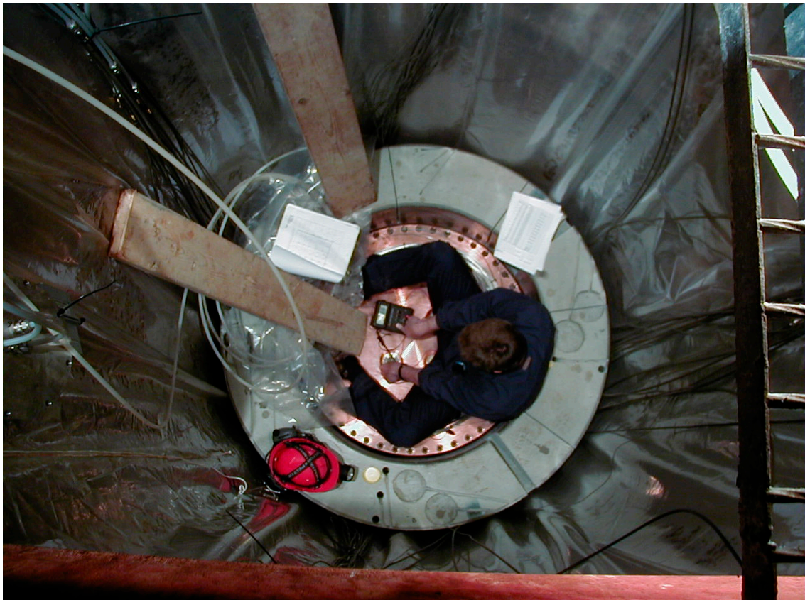
Figure 4-7 The three connectors on top of canister lid are checked.
