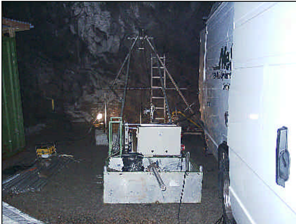
Figure 3-2. Photo of the winch system MKW-500 at the location of borehole no. KA2599G01.
