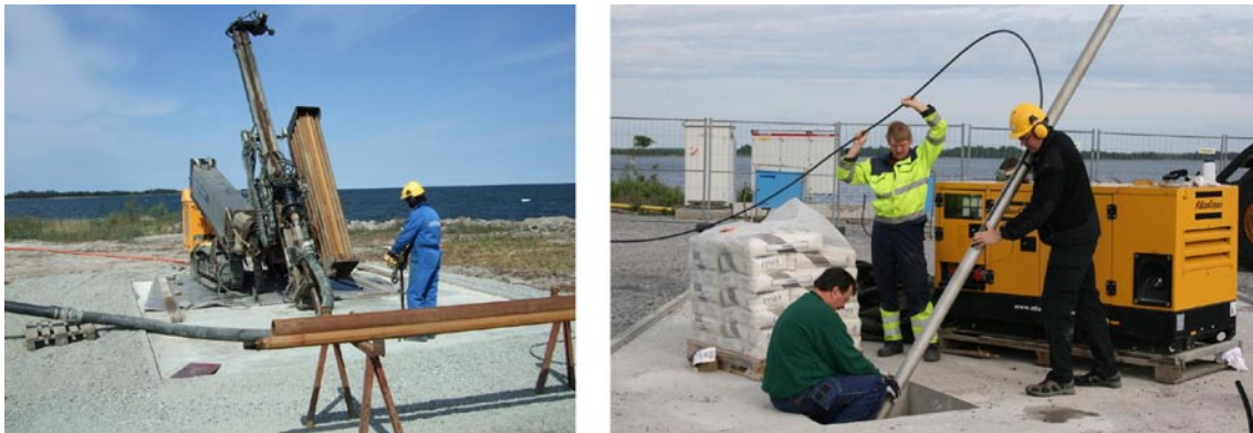
Figure 5-38. To the left the Nemek 407 RE percussion drilling machine is driving the casing through the overburden with the NO-X 115 technique. The photo to the right illustrates installation of an inner casing. Regarding KFR104 this was performed almost a month after completion of the percussion drilling. The section 0–8.73 m was supplied with an 88/77 mm stainless steel casing and the gap between the NO-X casing and the inner casing was cement grouted with use of the hose shown in the photo, from the bottom and upwards.
