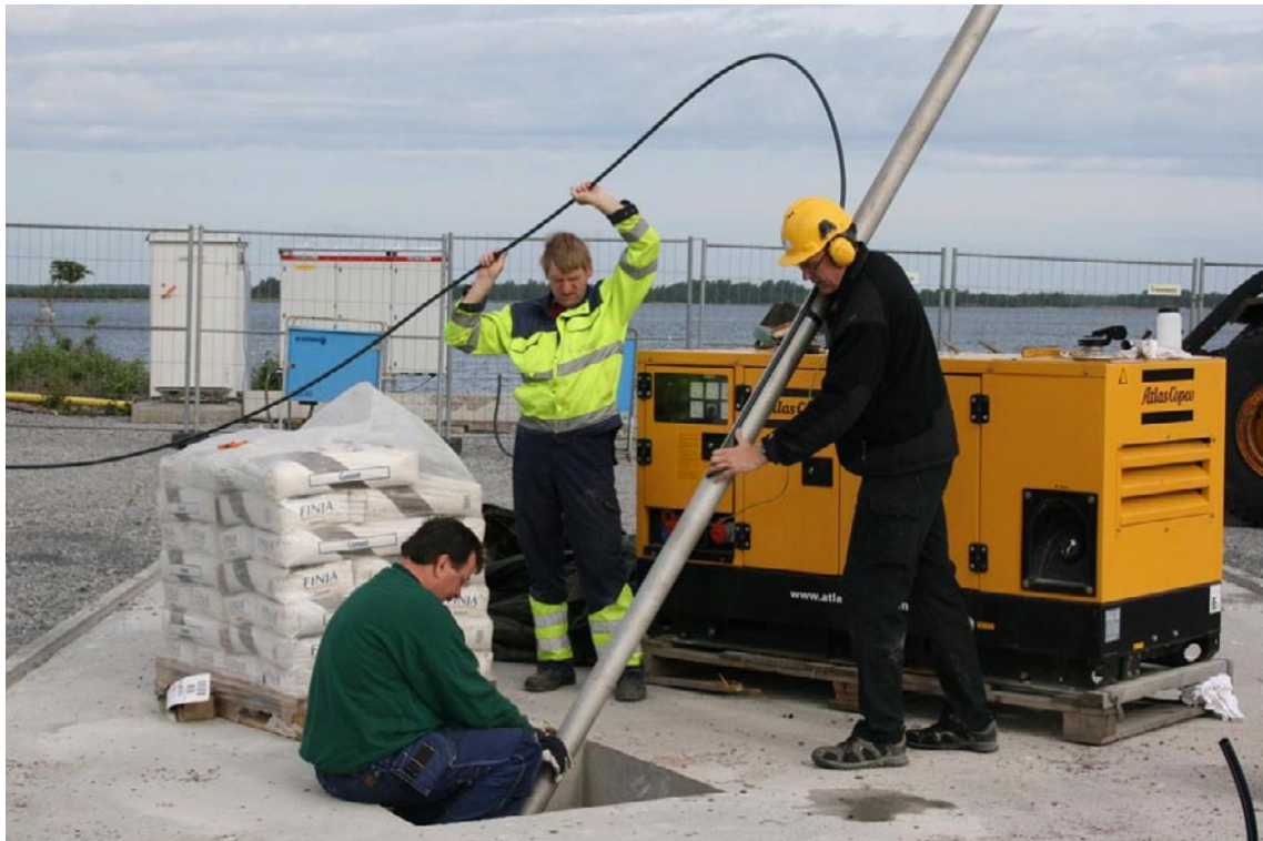
Figure 5-4. Installation of the inner casing was performed almost a month after completion of the percussion drilling. In KFR101 the section 0–13.72 m was supplied with an 88/77 mm stainless steel casing and the gap between the NO-X casing and the inner casing was cement grouted with use of the hose shown in the figure, from the bottom and upwards.
