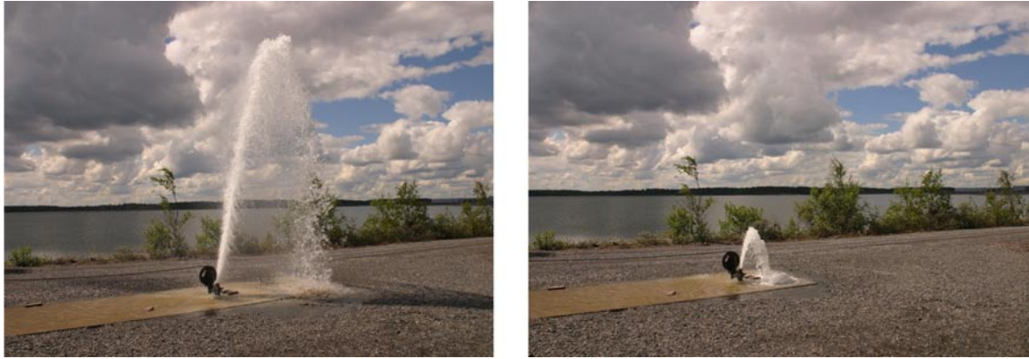
Figure 5-15. Nitrogen is forced through a hose to the bottom of the borehole. When the gas expands, the mixture of flushing water and drilling debris is lifted up from the borehole bottom. When the supply of nitrogen is closed, the gas- and groundwater outflow ceases. The groundwater level has to recover before further nitrogen flushing can begin.
