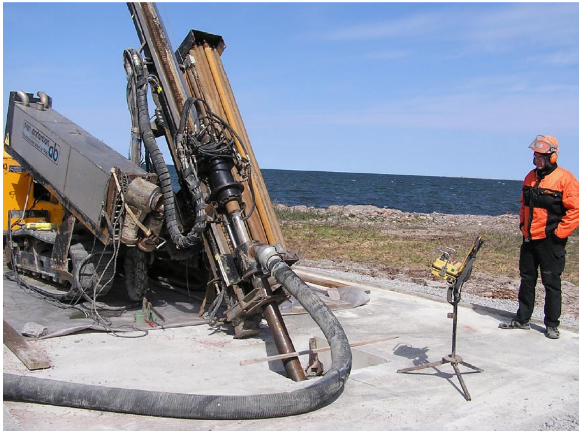
Figure 3-1. The Nemek 407 RE percussion drilling machine employed for pre-drilling and casing driving through the overburden with the NO-X 115 technique for the cored boreholes KFR101, KFR102B, KFR103 and KFR104.
