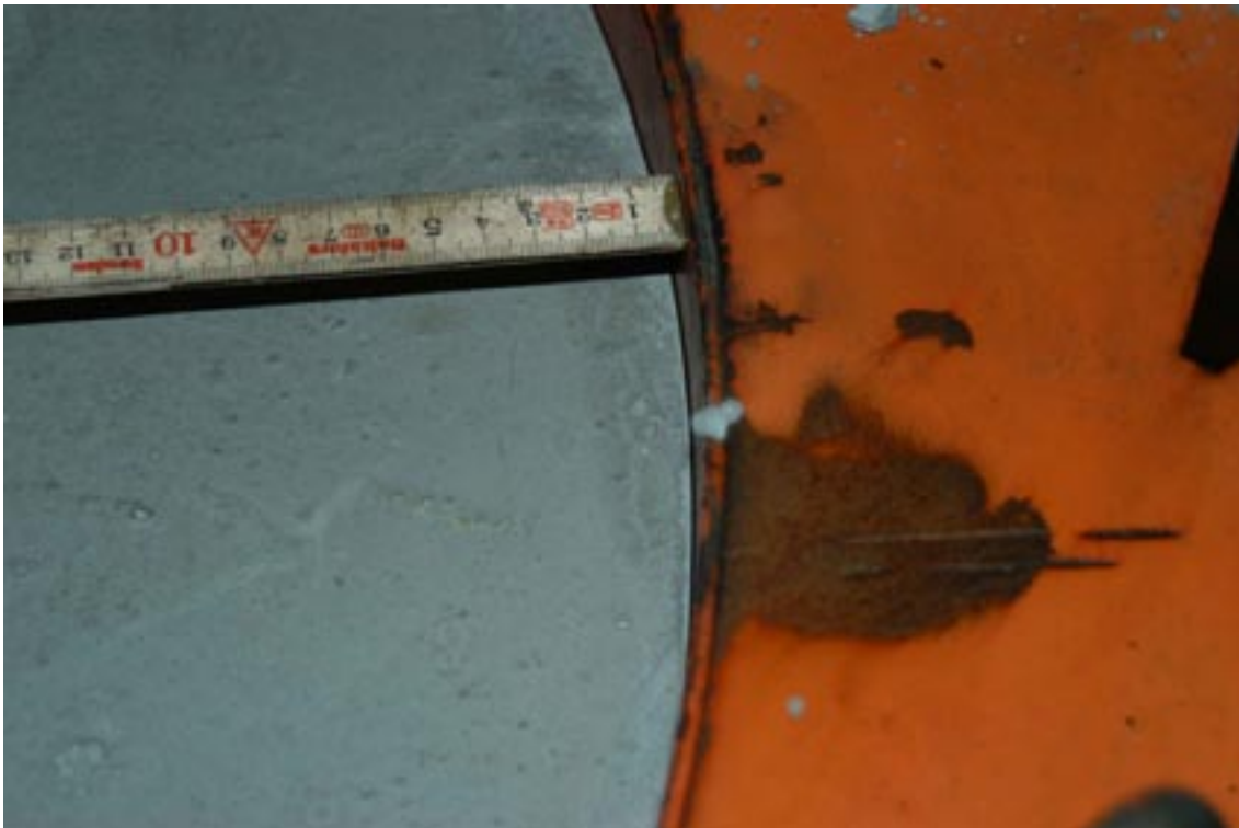
Figure 4-7. Gap between steel mould and concrete, one week after casting.
