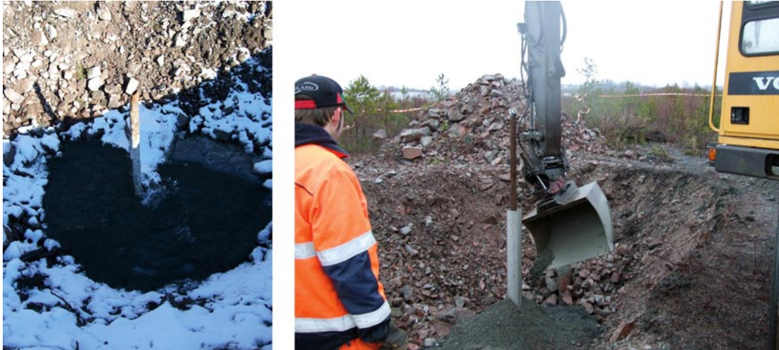
Figure 5-1. Left: The original and deformed casing of KFR27 was localised although it was covered with rock fill. Right: The casing has been extended above ground surface. An outer casing serves as a protective cover when the pit is re-filled with gravel.
