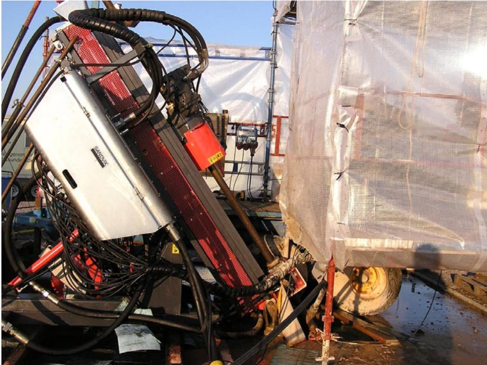
Figure 3-2. The more powerful rig Sandvik DE150 was used for drilling of the extended borehole KFR27.
