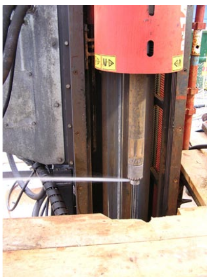
Figure 5-20. Flushing tool consisting of a nozzle mounted in the drill bit and designed to flush the borehole wall with high-pressurized water during simultaneous tripping and rotated in the borehole.
