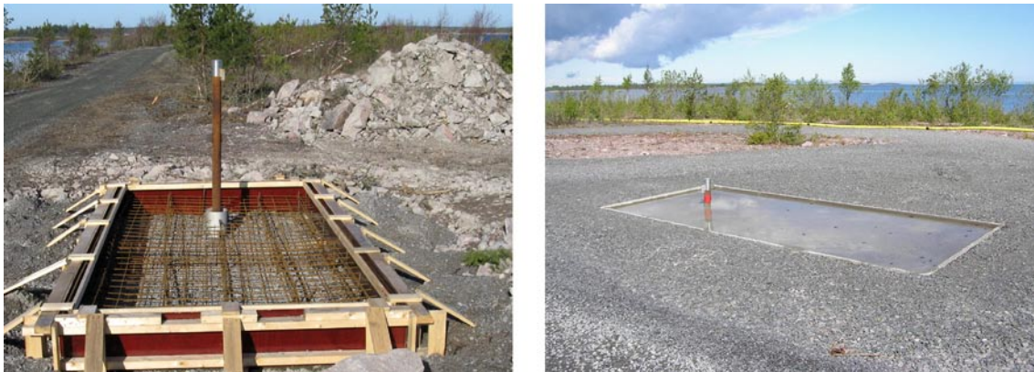
Figure 5-2. Left: A mould with reinforcing bars surrounding the borehole casing has been prepared for the concrete casting. Right: the drill site concrete platform is finished, filled up with gravel, and the casing is levelled for the drilling and measuring programme. Borehole KFR27 has been surveyed and the coordinates (according to the RT90-RHB 70 system) as well as the borehole inclination and azimuth are stored in Sicada, and the borehole is ready for investigations.
