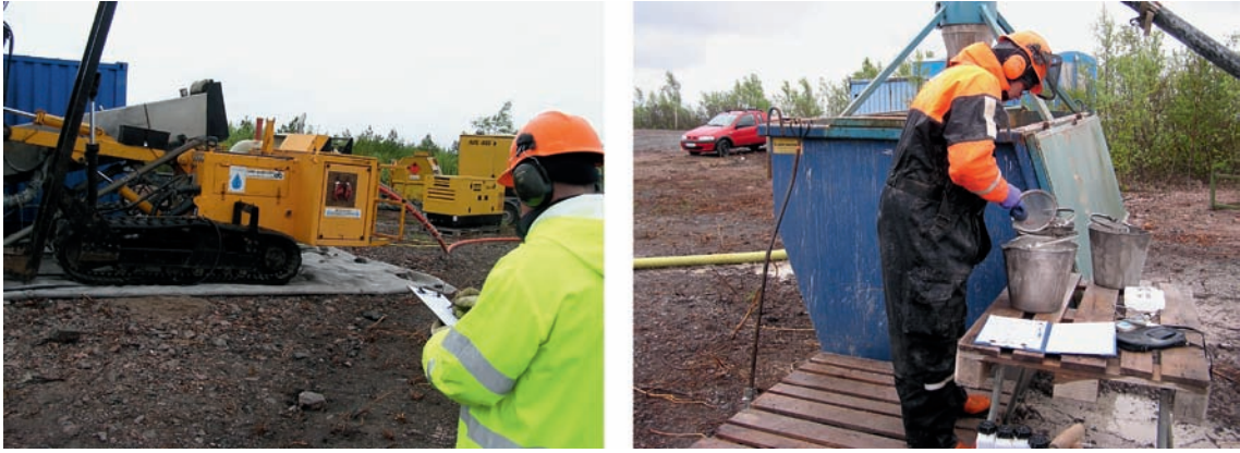
Figure 3-3. To the left, drilling penetration rate is manually measured with a stop watch, and to the right drill cuttings are sampled in a bucket of stain-less steel before placed in labeled pots.
