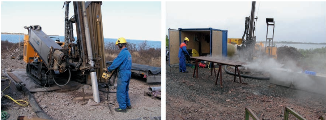
Figure 3-1. The Nemek 407 RE percussion drilling machine employed for drilling the percussion boreholes HFR101, HFR102 and HFR105. As the boreholes are of chemical type, all DTH-equipment was cleaned on-site with hot water.
