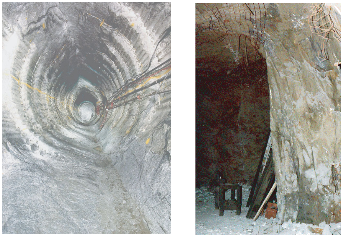
Figure 36: Examples of brittle failure (left photo - AECL's Mine-by circular test tunnel at the URL, right photo - rectangular shaped tunnel in a mine. Note the stress-induced fractures in the right photo. These have been removed in the Mine-by tunnel to show the v-shaped notch.
