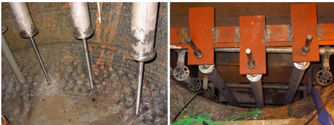
Figure 4-3. Lower (left) and upper (right) support for the vertical steel pipes. The pipes can be individually adjusted in height by using the nut the pipe is resting on at the lower support. Vertical movement due to thermal expansion is allowed through the upper support.
