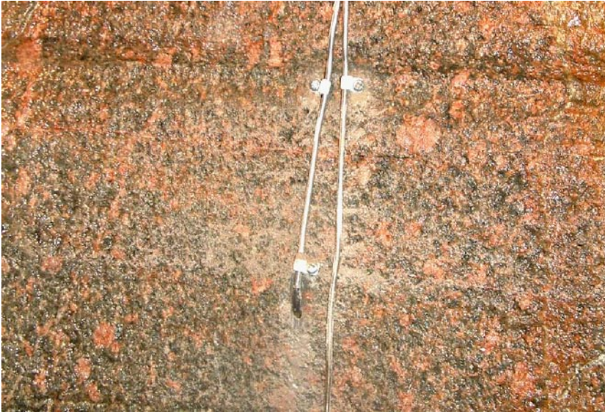
Figure 4-5. Placement of thermocouple in a small borehole drilled into the pillar wall.
