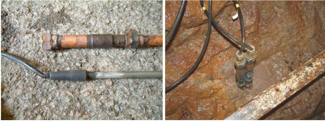
Figure 3-5. Left: photograph of heater element placed next to the protective copper tube. Right: heaters inside copper tubes installed in borehole which later was filled with sand.
