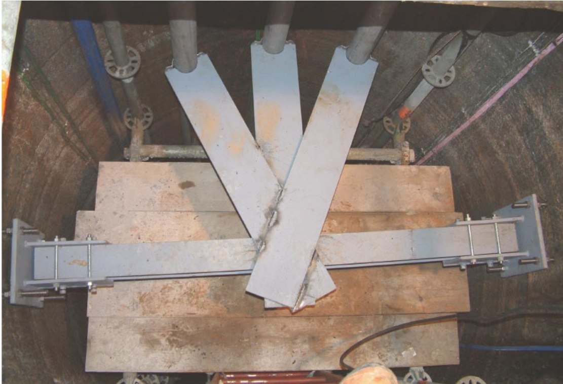
Figure 4-4. Photograph of the horizontal support of the vertical steel pipes close to the monitoring levels.
