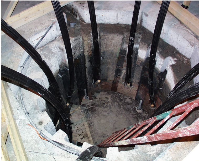
Figure 4-6 View of the top of Canister Retrieval Test hole showing the nine cable bolts and grooves between them for cables and pipes to pass the plug.
