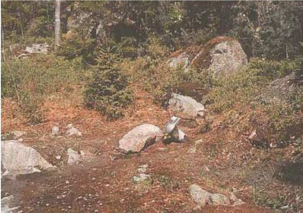
Figure 2-4. The dipping borehole 3 located in the ditch at the new parking lot at Boda. The borehole is directed into and under the cave area.
