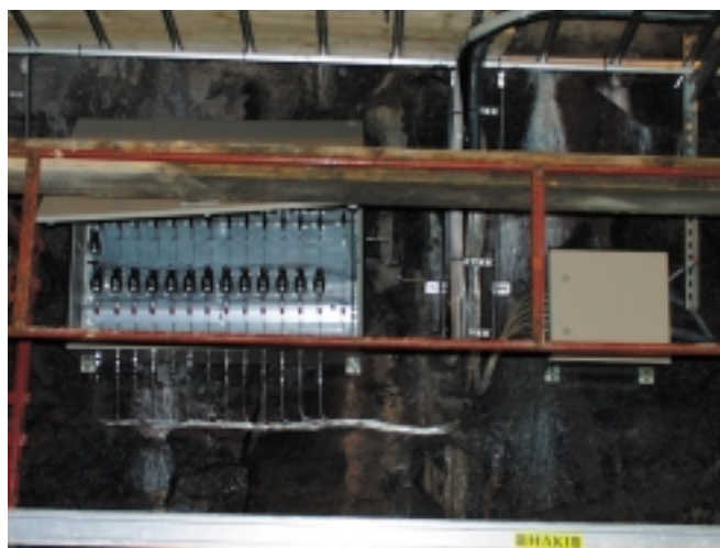
Figure 6-49. Valves box (left) and junction box at Demonstration drift.
