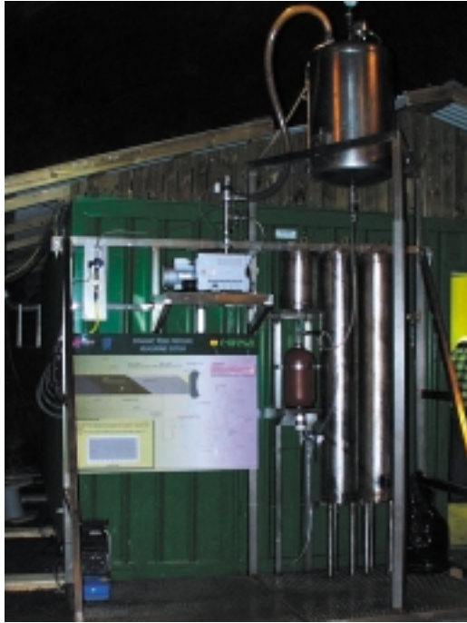
Figure 6-50. Measuring and control system (metallic structure outside control room).
