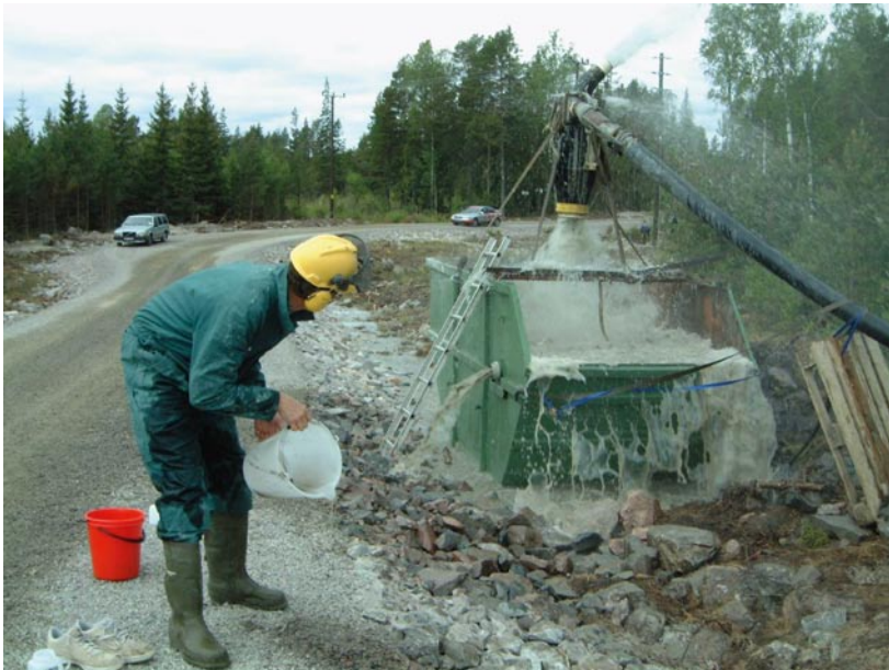
Figure 1-1. Picture showing the flushing of the percussion-drilled borehole HFM02 during completion. The estimated well yield at this instant exceeded 48,000 L/h.
