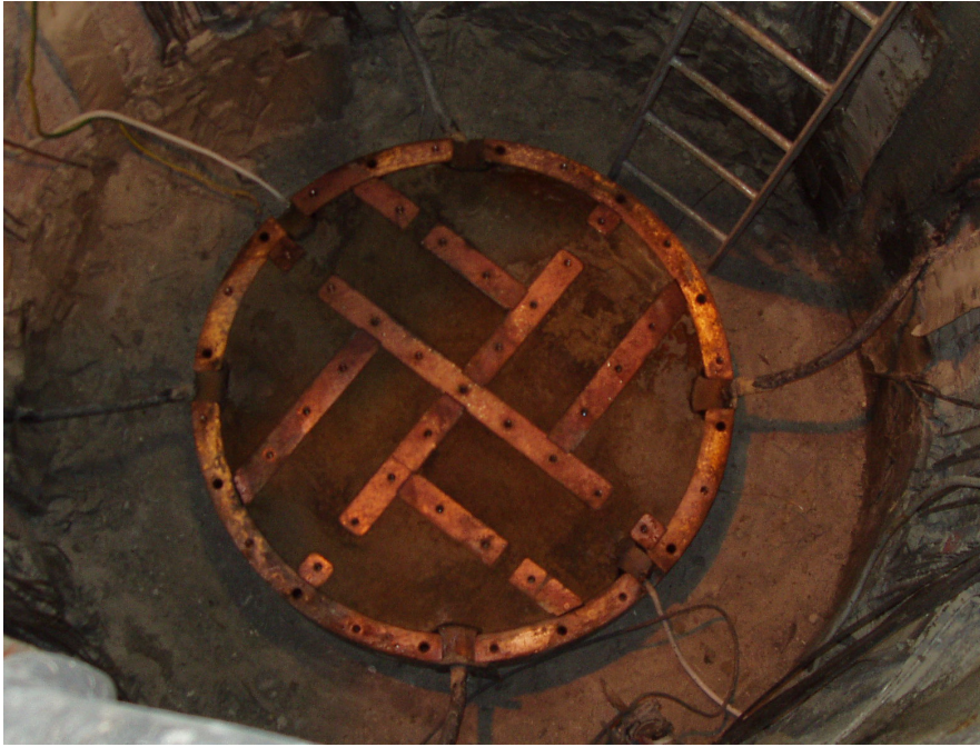
Figure 6-2. The upper lid is removed: The 30/70 mixture and the intermediate portions of copper are exposed.
