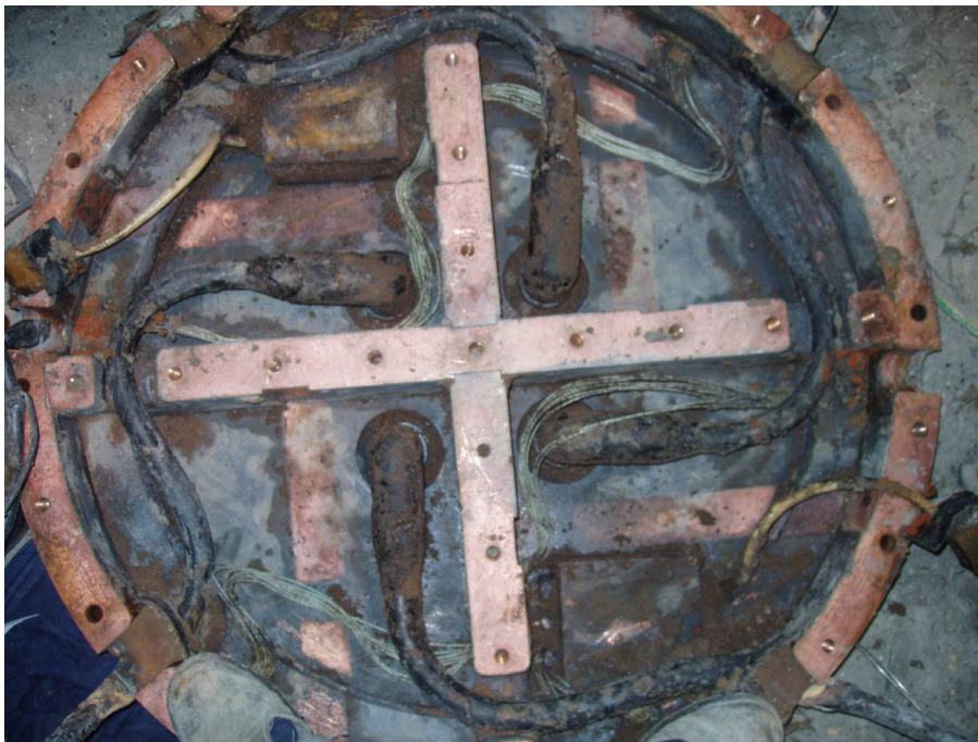
Figure 6-3. The cables and connectors on the top of the canister.
