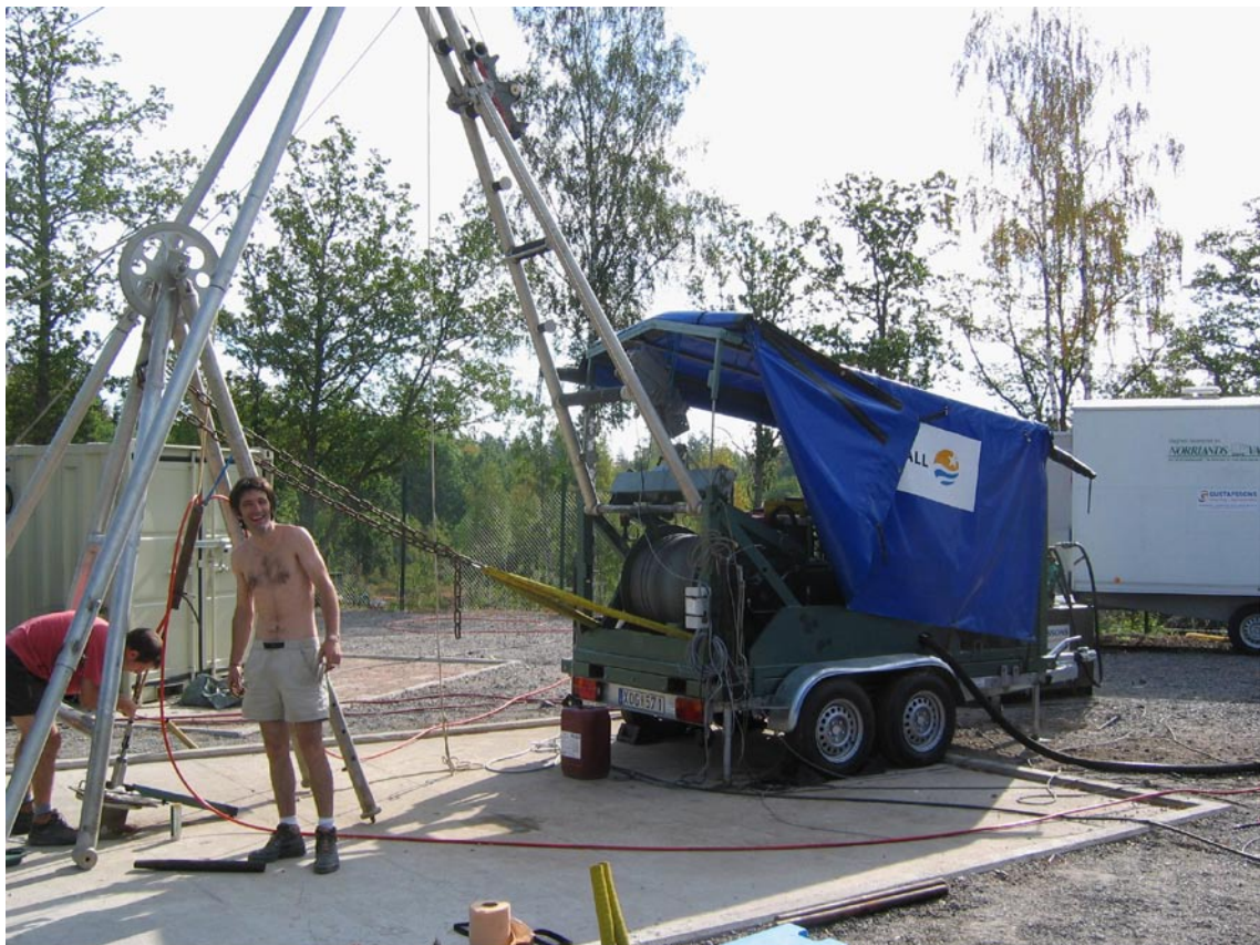
Figure 3-1. Photo of the upgraded MKW wireline unit of Vattenfall Power Consultant AB during operation in borehole KLX12A.
