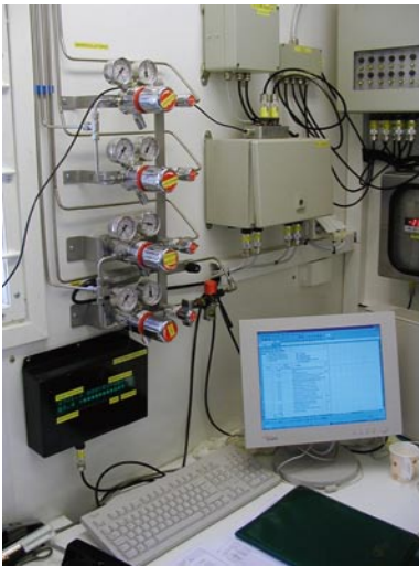
Photo 3. Computer room, displays and gas regulators.
