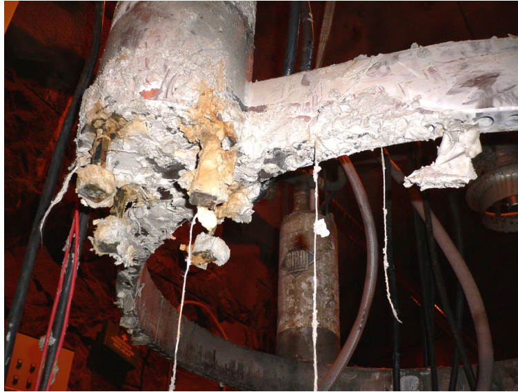
Image 6-2. Suction nozzle clogged by rags, strings and bentonite clay. (Photo: Bo Nirvin, SKB).
