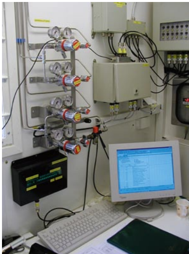
Photo 3. Computer room, displays and gas regulators.
