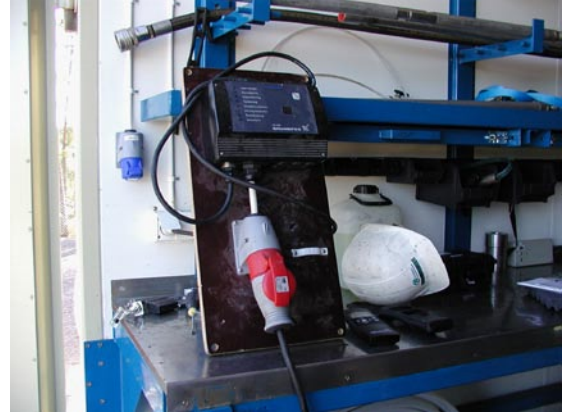
Photo 8. Control board of the pump with remote control.
