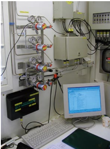
Photo 3. Computer room, displays and gas regulators.
