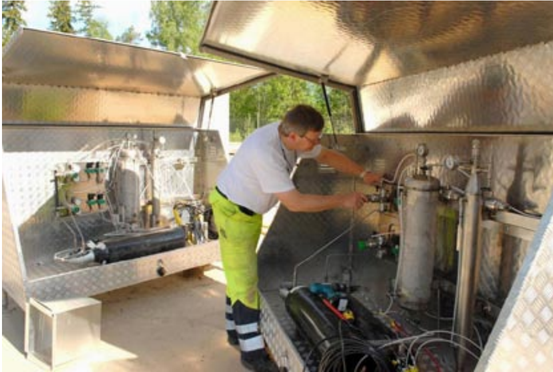
Figure 4-14. Interior of two housings used as borehole collar shelters after installation of groundwater level monitoring equipment in percussion drilled boreholes.
