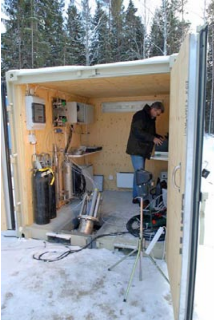
Figure 4-13. Interior of container used as borehole collar shelter after installation of groundwater level monitoring equipment in a core drilled borehole of telescopic type.
