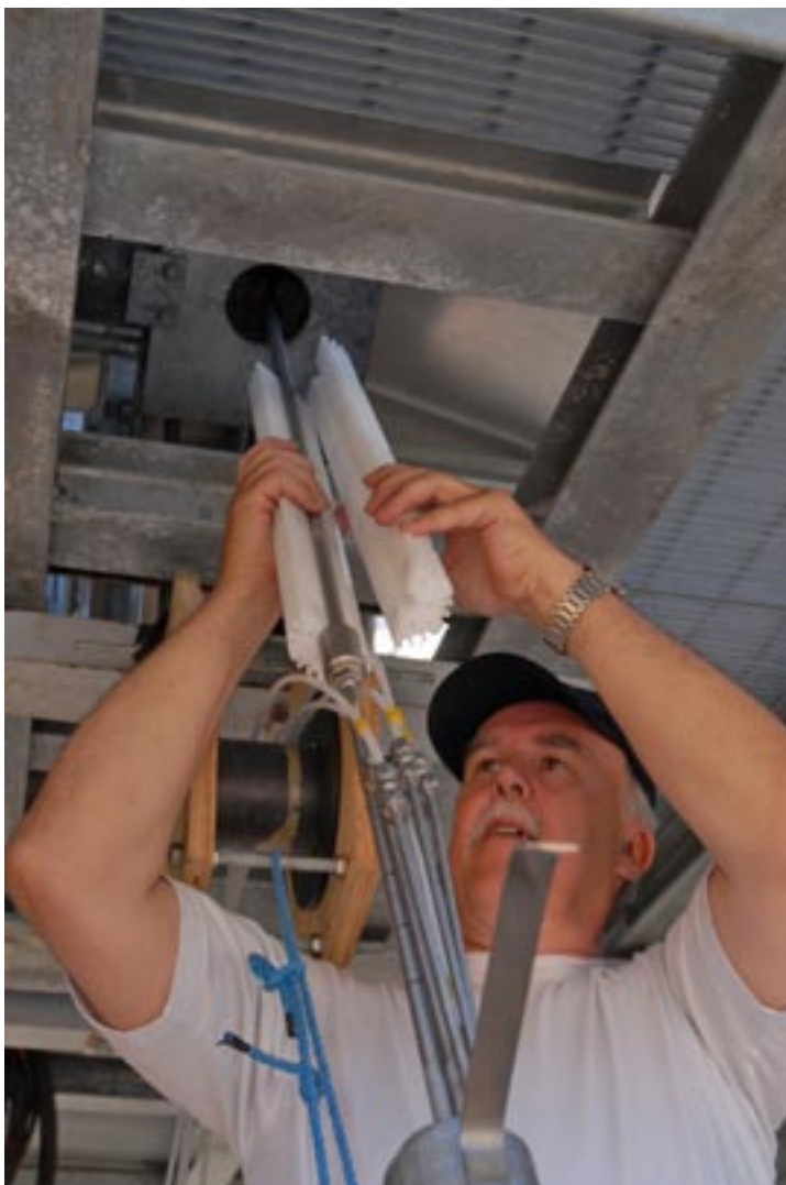
Figure 4-12. Installation of equipment for groundwater level monitoring in a core drilled borehole.
