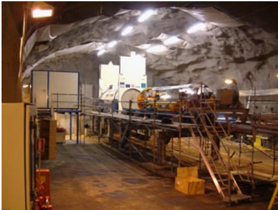
Figure 4-23. The KBS-3H deposition equipment in the niche at –220 m level at Äspö HRL.
