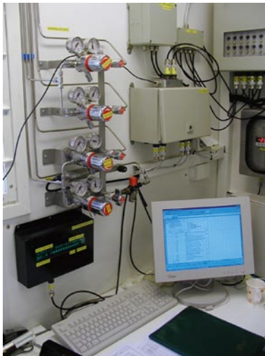
Photo 3. Computer room, displays and gas regulators.
