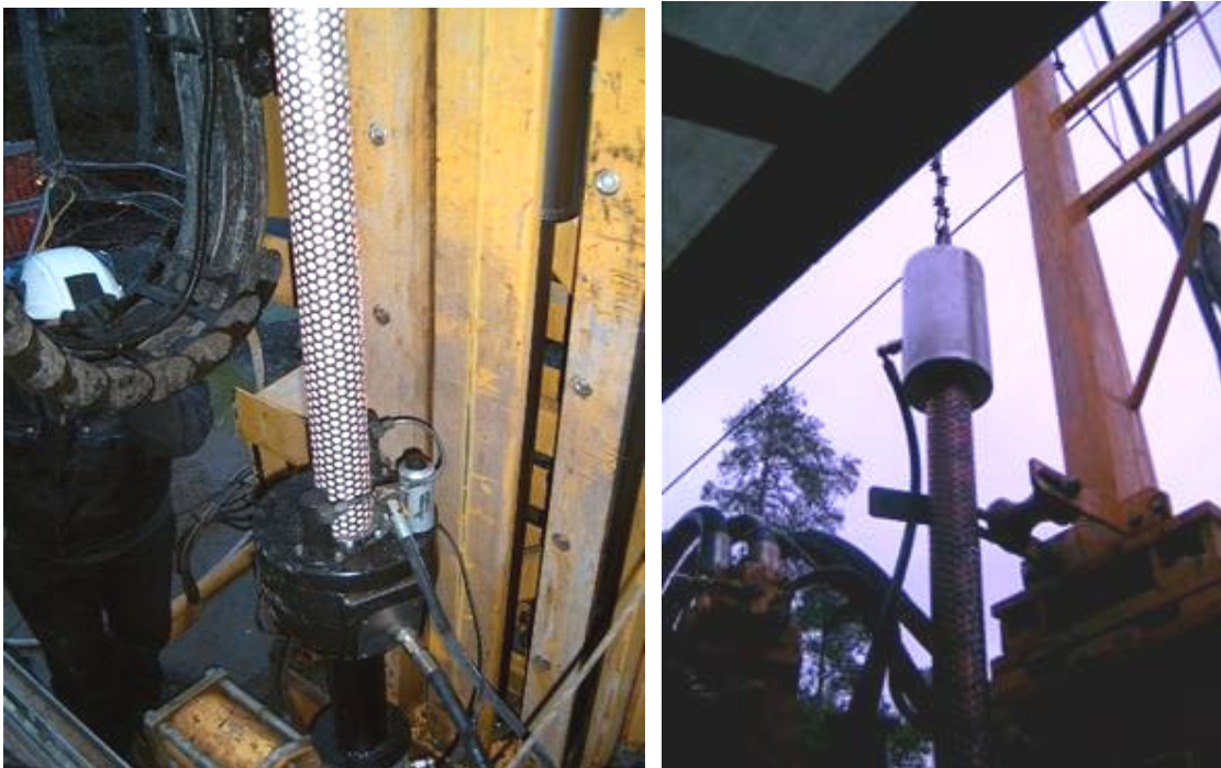
Figure 2-6. Left: Jointing of two 2.5 m long units. Right: Hydraulic equipment for handling the copper tube during installation.
