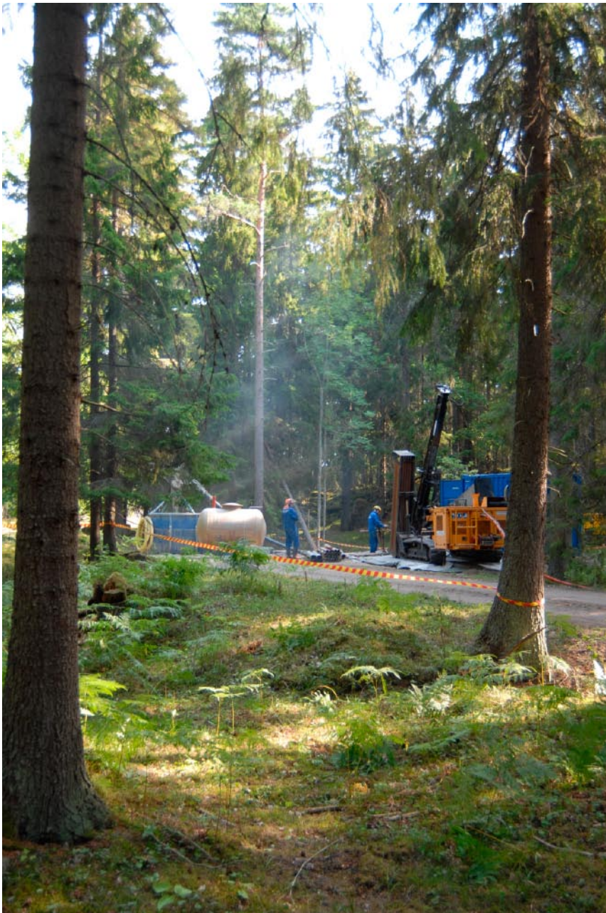
Figure 3-1. The Nemek 407 percussion drilling machine employed for drilling the percussion boreholes HFM36, HFM37 and SFM0109 at drill site DS12. Here during drilling of HFM37.
