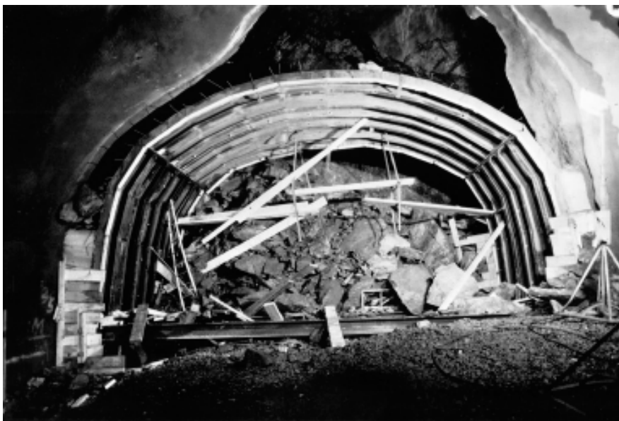
Figure 4-13. Rockfall in Tunnel 3 at the intersection with the Singö deformation zone. Steel sets were used for temporary support and for formwork for a cast concrete arch from /Carlsson et al. 1985a/.
