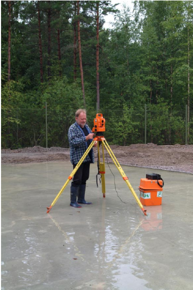
Figure 4-1. Gerry Johansson from Geocon preparing the lining up of the drilling machine.
