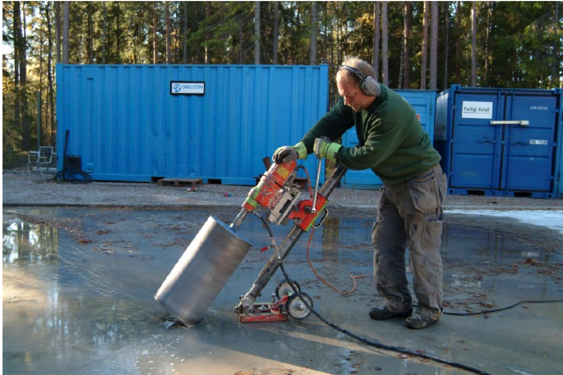
Figure 4-2. Special drilling equipment was used for making a hole through the concrete slab to prevent reinforcement bars to damage the drill bit when drilling KFM09B.
