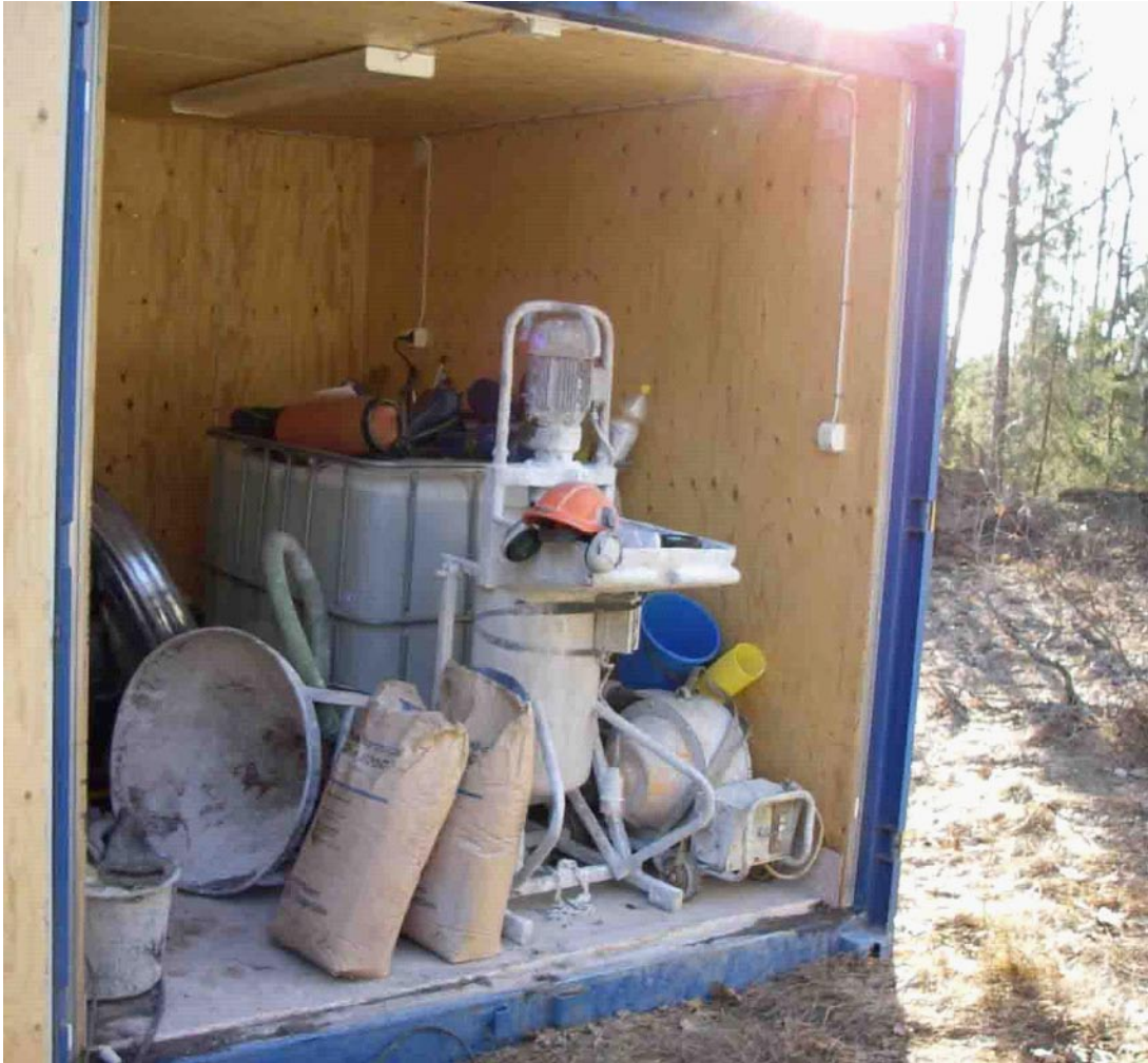
Figure 4-5. Mixing station for the concrete slurry. The slurry is pumped from the mixing station through the tremie pipe and packer into the borehole.
