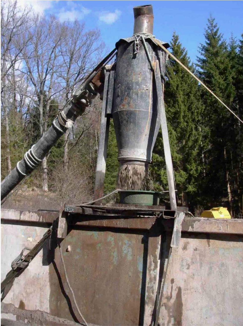
Figure 4-6. Return water from drilling (HLX38) is led to a settling container. The cyclone for directing the cuttings to the collecting sieve can be seen fastened on top of the container:
