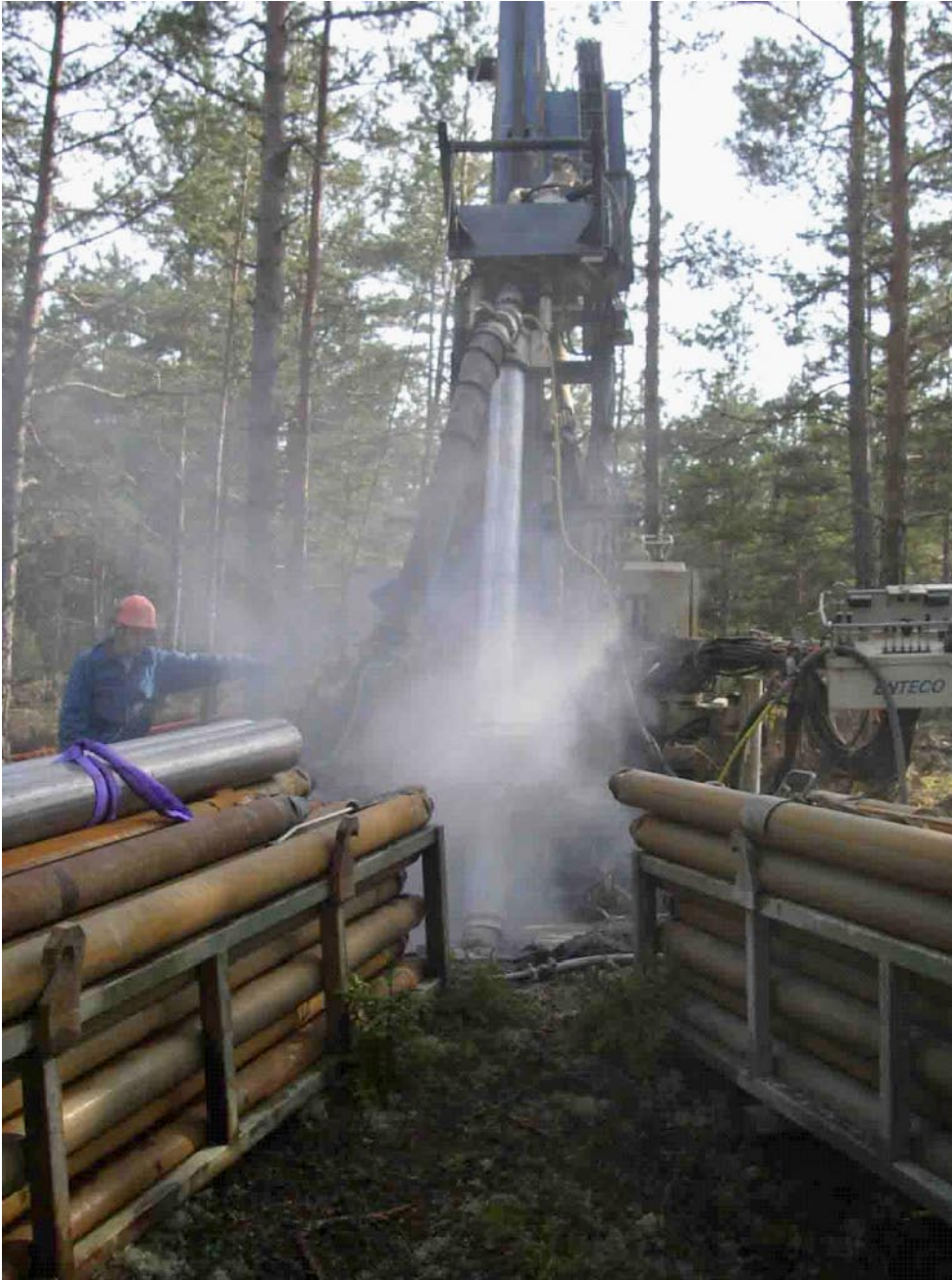
Figure 4-1. Starting up the casing drilling with TUBEX 140 in HLX40. The stainless steel casing rests on the excentric drill bit.
