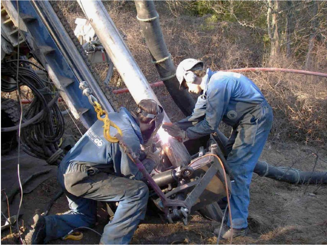
Figure 4-2. Welding of casing in HLX38. The sections of casing are welded together in order to provide a watertight seal to the surrounding soil and water.
