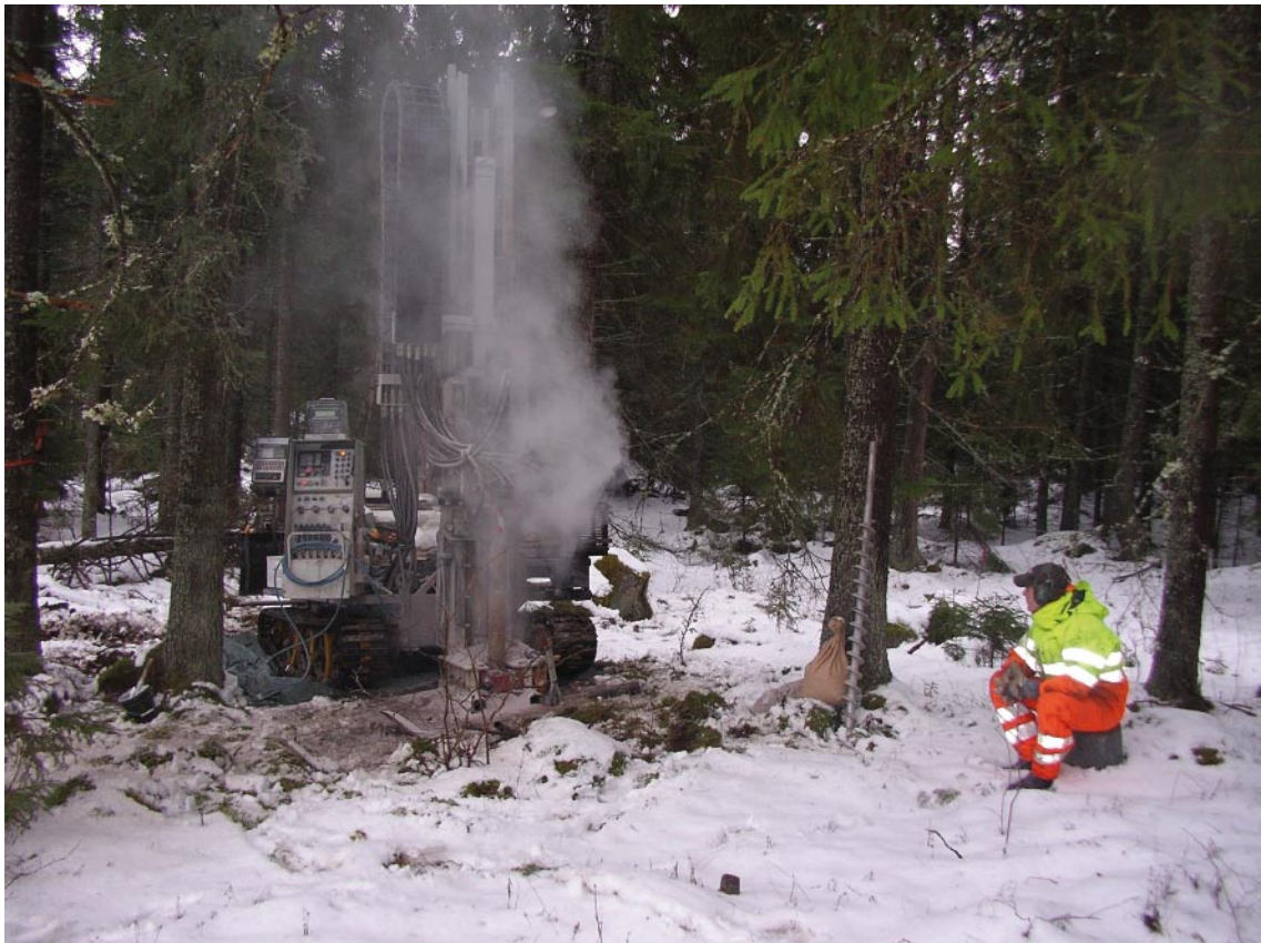
Figure 3-1. Installation of groundwater monitoring well SFM0105. A GeoMachine GM 100 GTT drilling rig with an 8-bars Dynaset air compressor was used for installation of all groundwater monitoring wells and pumping wells on ground with good bearing capacity.
