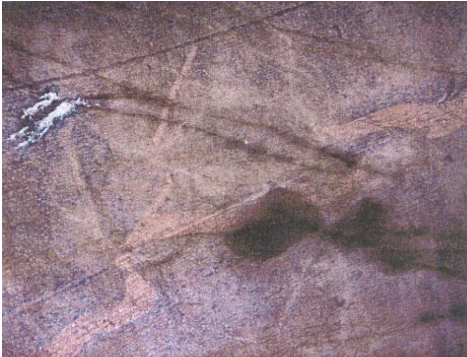
Figure 2-55. View of one of the bored tunnels at Äspö showing conductivity along discontinuous fractures. These fractures may be linked via a parent fracture (see Figure 2-53) or via small cross fractures which, in this example, do not outcrop on the tunnel wall.
