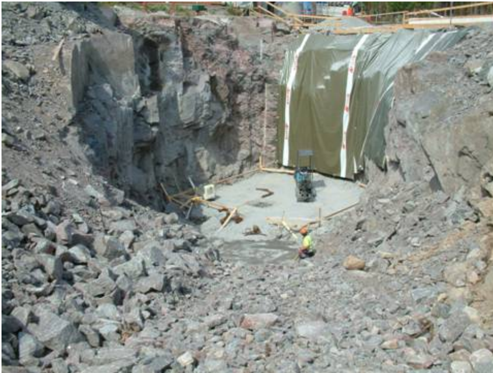
Figure 3-1 The excavated cavity in the rock was prepared with base course gravel.
