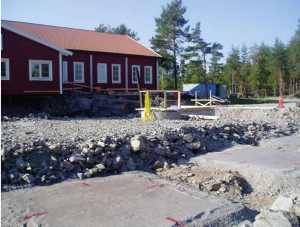
Figure 3-2 The upper parts of the two deposition hole constructions can be seen above the backfilling material.
