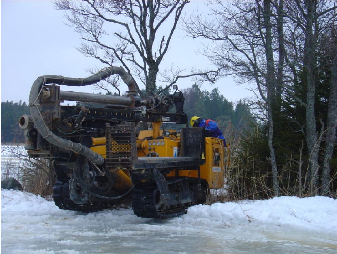
Figure 3-2. The Nemek 407 percussion drilling machine employed for drilling the percussion boreholes HFM30, HFM31, HFM32 and HFM38. Here establishing for drilling HFM32 at a small island in lake Bolundsfjärden.
