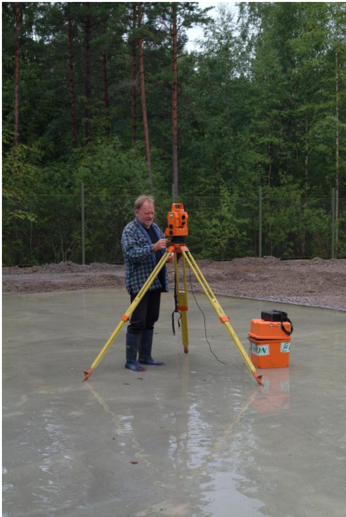
Figure 3-5. Strike and dip for the borehole is measured with a GPS and a compass. The borehole is finally positioned and measured for strike and dip with a theodolite instrument.
