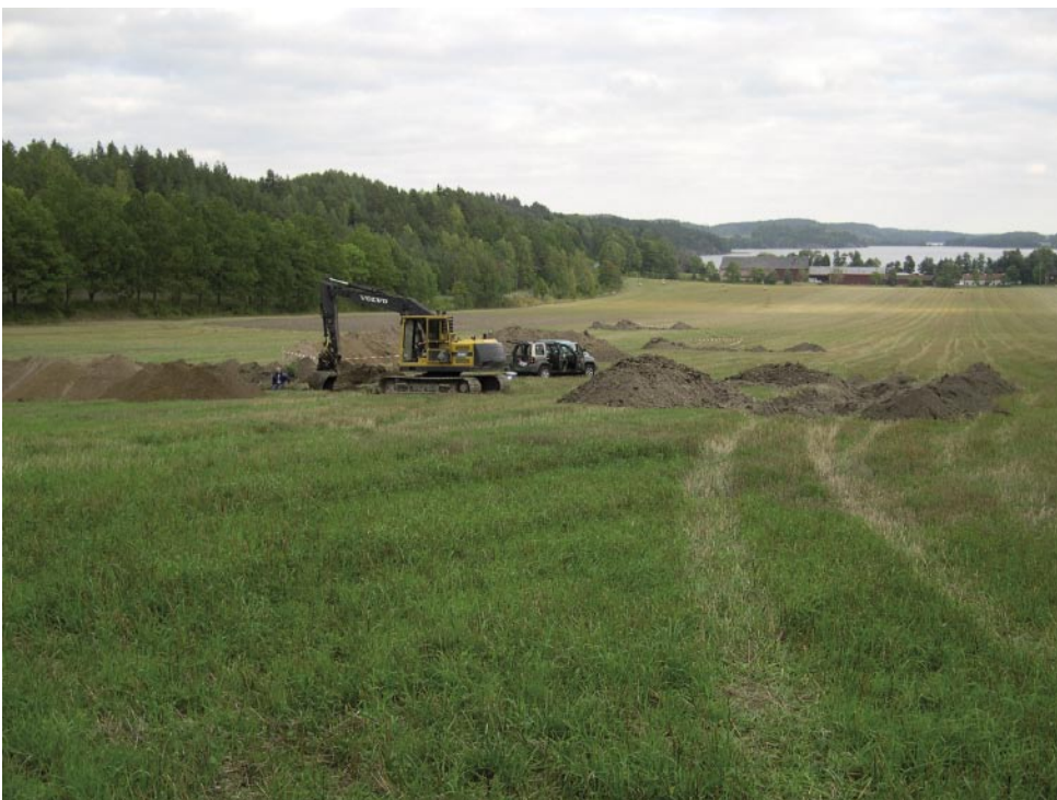
Figure 4-2. Typical excavation site in gently sloping, cultivated ground at Ukna (E13 in Figure 1-1), centrally located in the Uknadalen valley. The pits in the distance (see earth-mounds) contained glacial clay to a depth of at least 3.5 m and were not considered appropriate for investigation, while the trench under excavation contained thick deposits of loosely packed glaciofluvial sand and silt.
