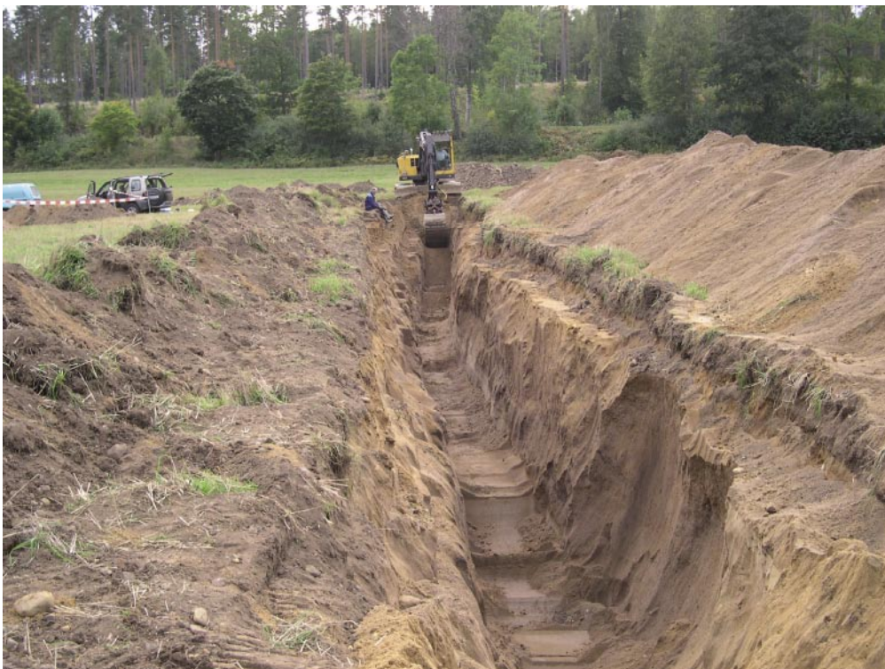
Figure 6-2. Trench dug in loosely packed glaciofluvial sand at Ukna (E13 in Figure 1-1). The excavation site is centrally located in the rather impressive Uknadalen valley, one of the few morphological features in the investigation area that might conceal major recent fault movement from detection (cf. Figure 4-2). Deformational features interpreted as caused by sliding and debris flow were met with but no indication of liquefaction whatsoever was noted in the thick deposits of loosely packed sand.
