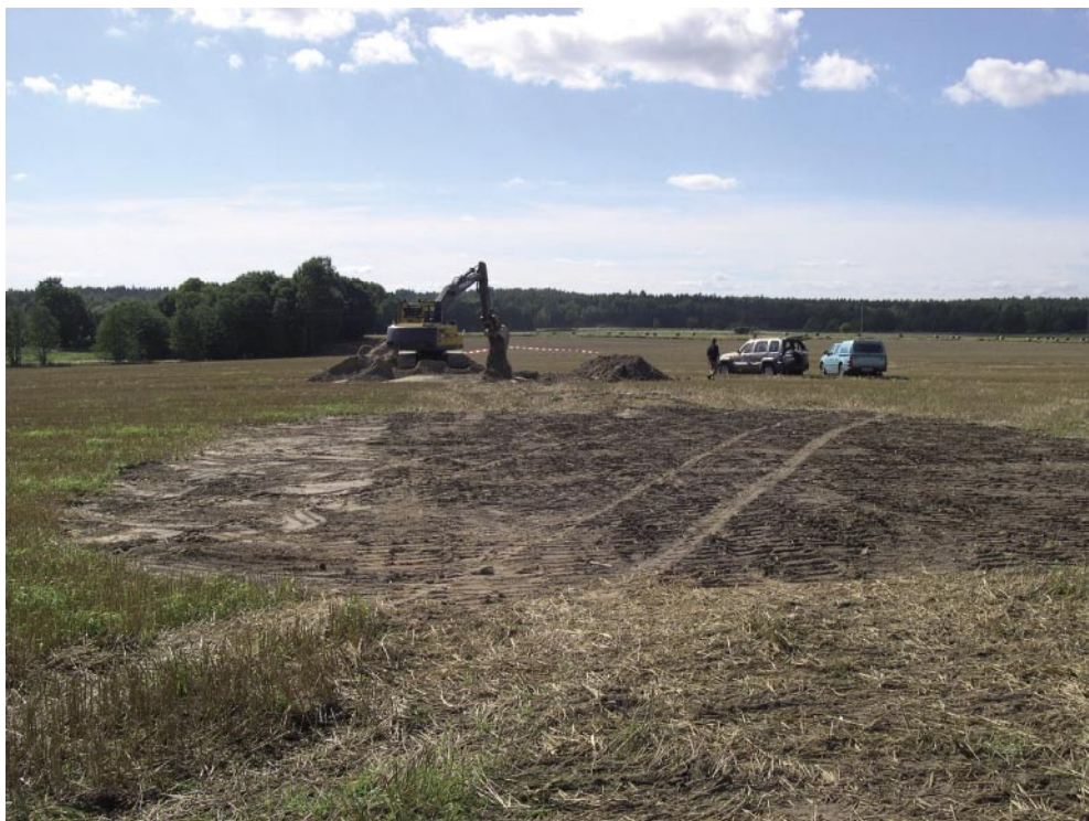
Figure 4-4. After documentation the trenches were filled in and, by returning the former topsoil to the ground surface, the cultivated ground was restored. Excavation site E7 at Staby.
