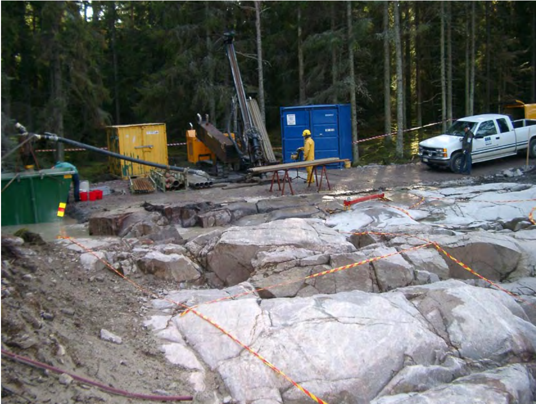
Figure F-3. The Nemek 407 percussion drilling machine in operation at drill site 5. Water and drilling debris is discharged to the container to the left. The fractured bedrock is seen in the foreground.
