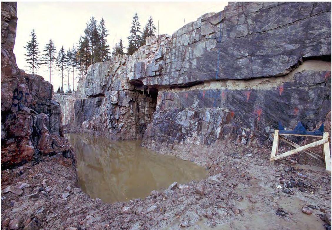
Figure 5-1. A shaft wall of a storage basin for industrial water under construction at Forsmark. This was one of several excavations investigated by /Carlsson 1979/ during the period when the nuclear power plants and auxiliary facilities were constructed. The system of extensive, horizontal and subhorizontal fractures can be seen, as well as steeply dipping fractures. The outstanding, horizontal fracture is c 0.5 m wide and filled with sediment. Photo Göran Hansson/N.
