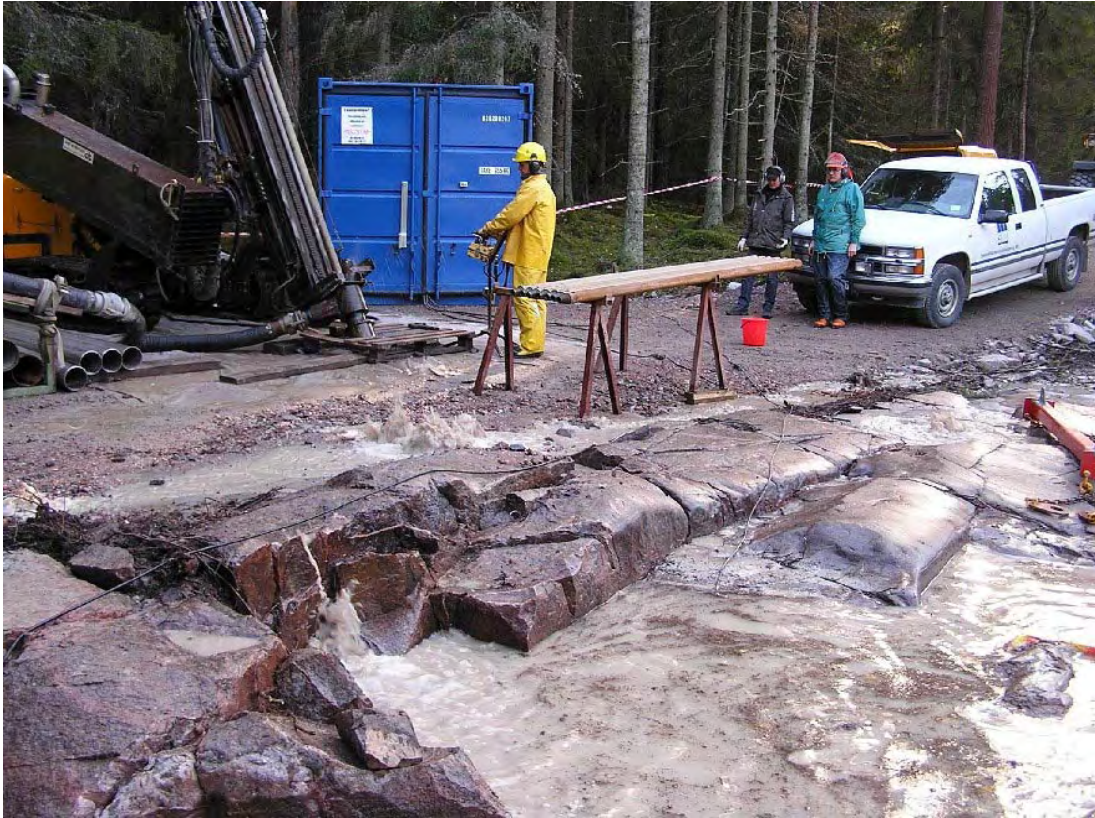
Figure F-6. When drilling HFM14, flushing water was flowing in open fractures, from the borehole to surface.
