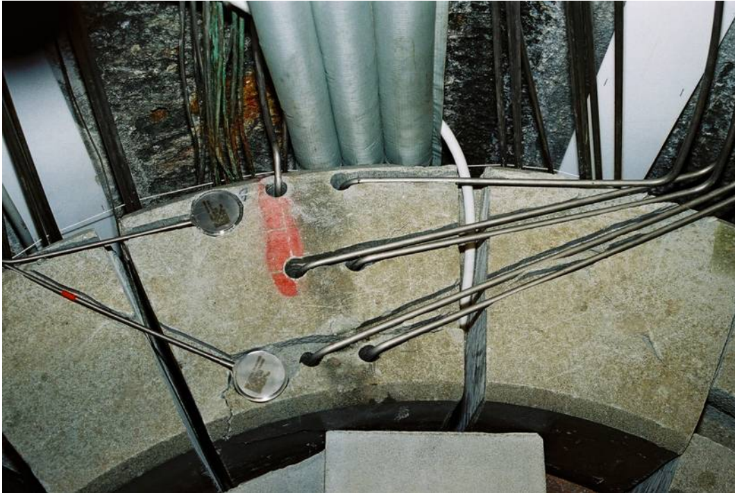
Figure 5.6-3. Picture of the upper ring (R10) taken after placement of the canister and installation of the instruments. The big radial slots are for the fibre optic cables on the canister surface (left) and the cables from the thermocouples and strain gauges in the canister. The two pucks are total pressure gauges and the six holes contain relative humidity sensors.
