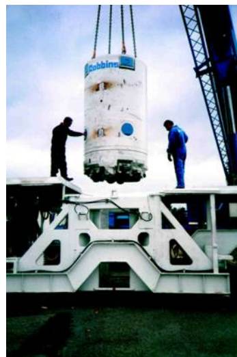
Figure 5-15. TBM-type equipment (Robbins) used for boring of vertical deposition holes with 1.8 m diameter and 8 m depth.
