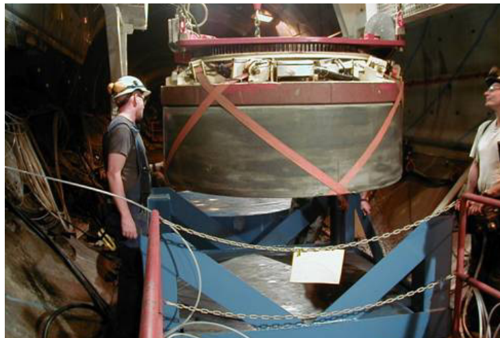
Figure 3-12. Application of a 2 Mg buffer block of bentonite in a deposition hole. (SKB)
