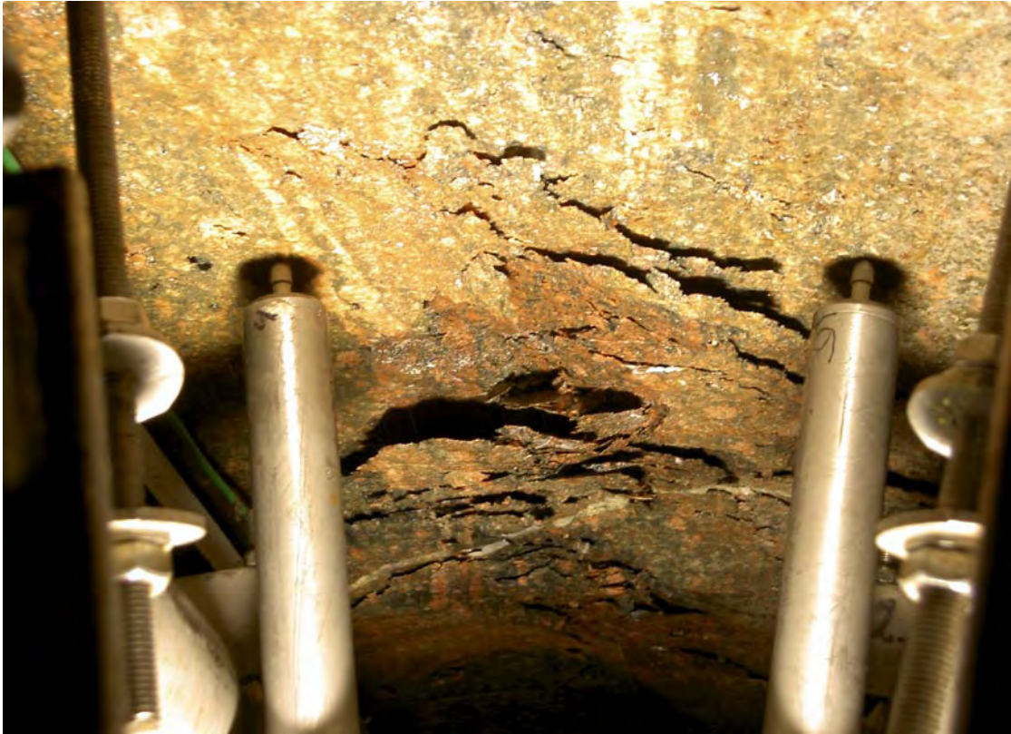
Figure 3-2. Photograph of spalling precisely as it has reached one instrument level.
