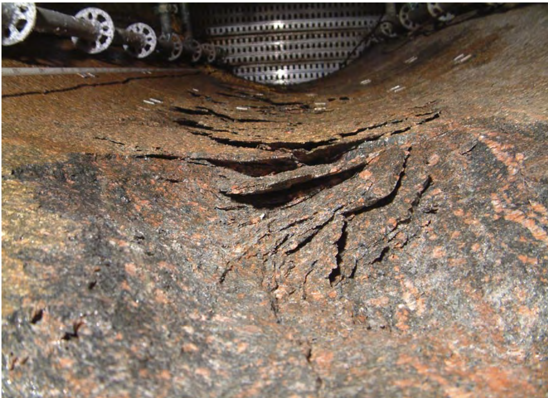
Figure 3-3. Photograph of the pillar wall as the slabs are being removed from the bottom and up.
