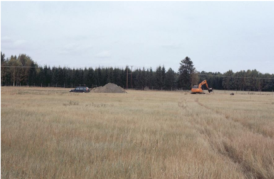
Figure 4-5. Typical excavation site in very gently sloping ground along the Börstil esker. Kråkmötet (E4 in Figure 4-1) after opening of a first test pit.
