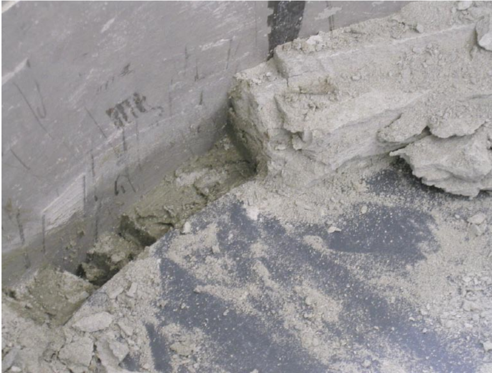
Figure BB7-4. Picture showing the PVC dummy and the slot which at excavation was filled with bentonite. As shown only a very small part of the bentonite block took part in the sealing. About 5 cm radial from the edge of the dummy the bentonite is dry.
