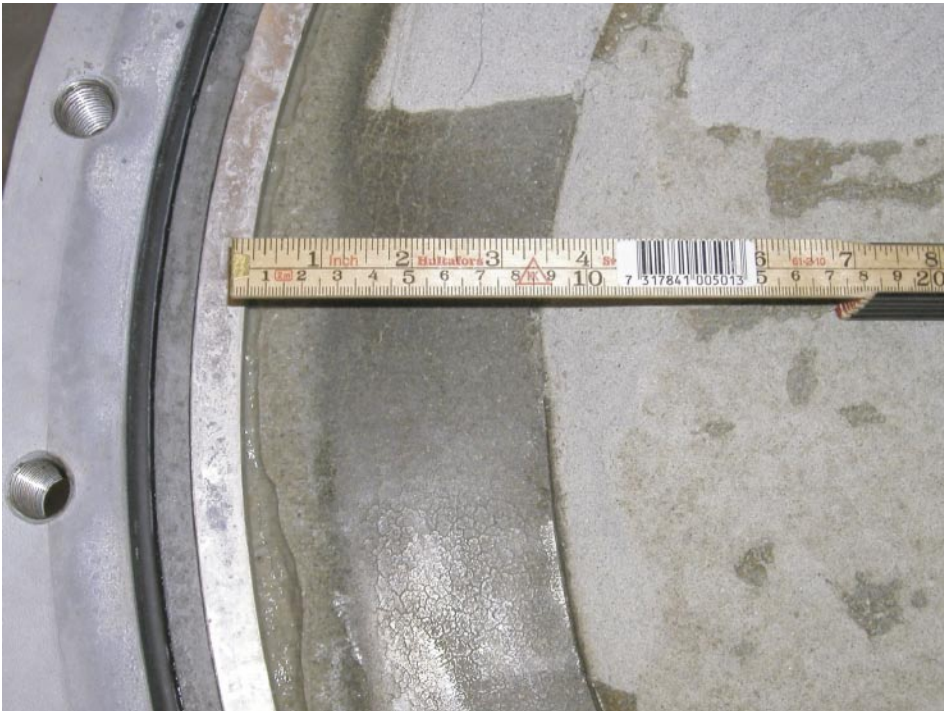
Figure BB2-6. The wetting and sealing of the zone behind the collar ring.
