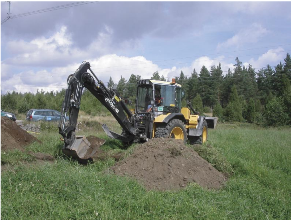
Figure 3-3. The tractor excavator at a trench in the local model area near Laxemar (PSM005410).
