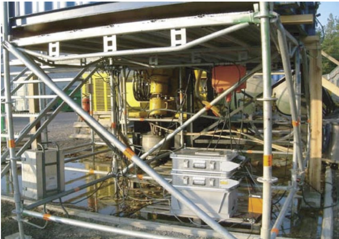
Figure 4-3. The CR23 logging unit for parameters “air-pressure” and “electrical conductivity”.
