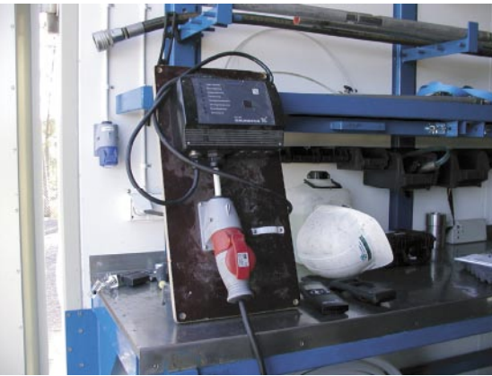
Photo 8: Control board of the pump with remote control
