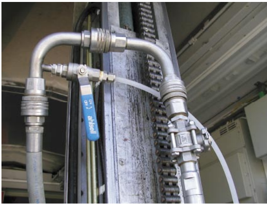
Photo 7: Top of test string with shunt valve and nylon line down to the pump basket
