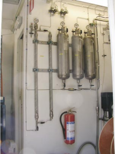
Photo 4: Pressure vessels for test valve, packers and injection.
